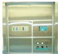
Medical gas unit
